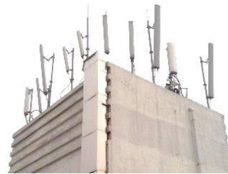
Fig. 1. Base-station antennas on a building.
