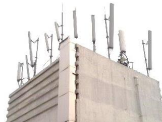
Fig. 1. Base-station antennas on a building.
