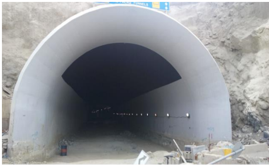
Fig. 7. Arched tunnel for cars, flat base ( L ) = 14m, radius a = 7.3\text{m} , and height at center = 10.35m.
